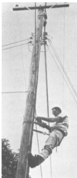
System technicians "tap" a cable drop from the main trunk into the subscriber's home.
