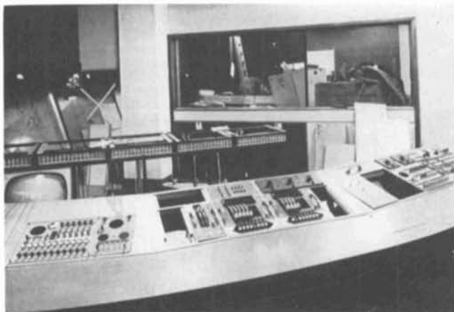
Studio 3's vision control room: the main production desk during installation.
