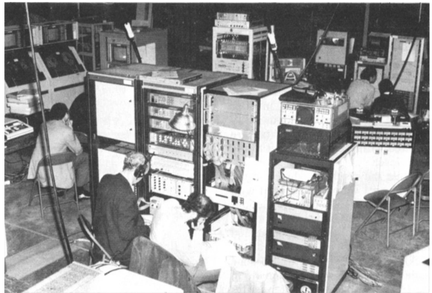
Figure 4. Central equipment cluster. The rack on the left contains the switching matrices. To the right is the rack with test signal generators, the UltiMatte, sync generator, and zone plate generator. Further right is the rack with the analog decoders at the top, processing amplifier, digital patch panel, and routing switcher control. The rack on the extreme right has converters for analog RGB to digital components and for digital components to analog RGB plus an encoder for digital components to analog NTSC.
