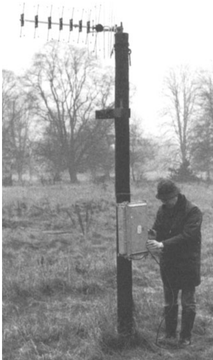
Figure UK-7. Mock-up of a small UHF re-broadcast television transmitter of the type that will be used by "self-help" groups in the United Kingdom.
