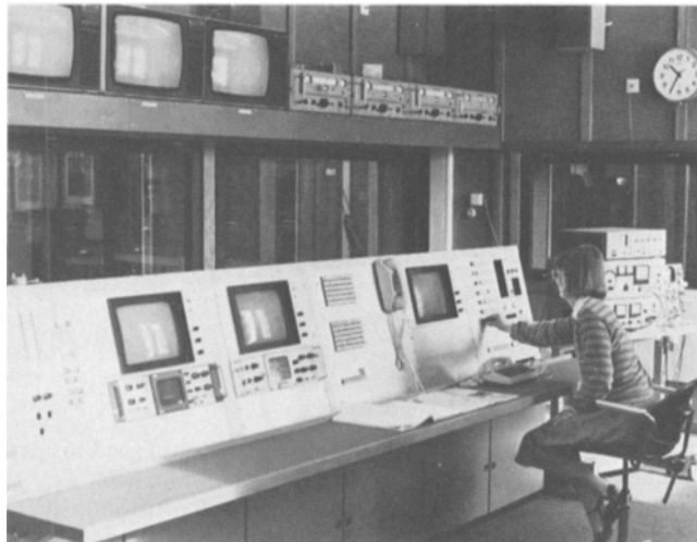
Figure F-4. Control room of the Tampere transmitting station.
