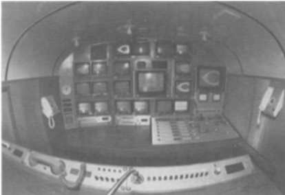
Rack and technical equipment area.
