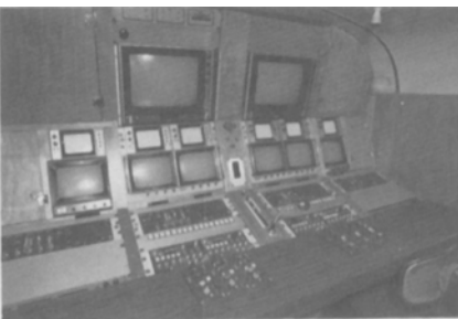
Camera control area.
