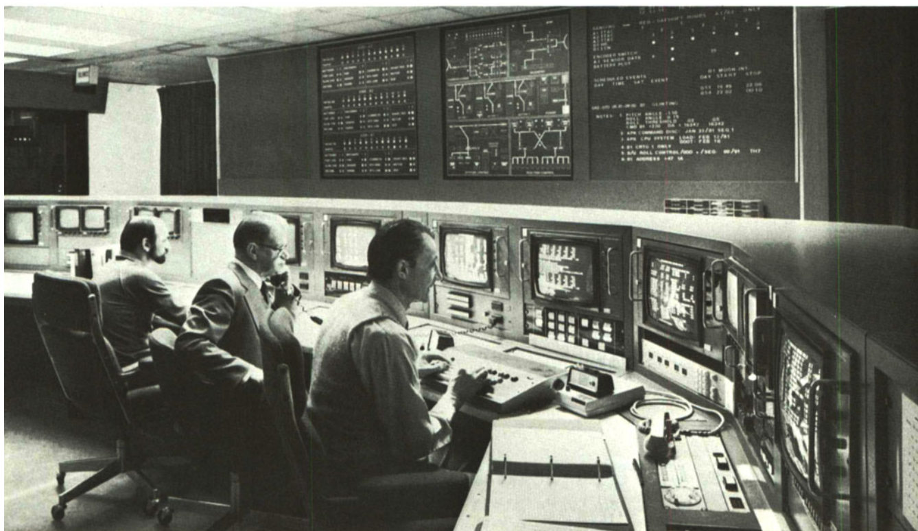
Satellite Control Centre at Telesat Canada, Ottawa, Ont., shown to members and guests at the Ottawa Section meeting, January 20.
