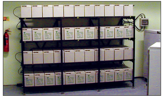
Emergency battery room. Warner, Islington
