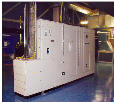
Electrical intake equipment, Ster Century, Romford.
