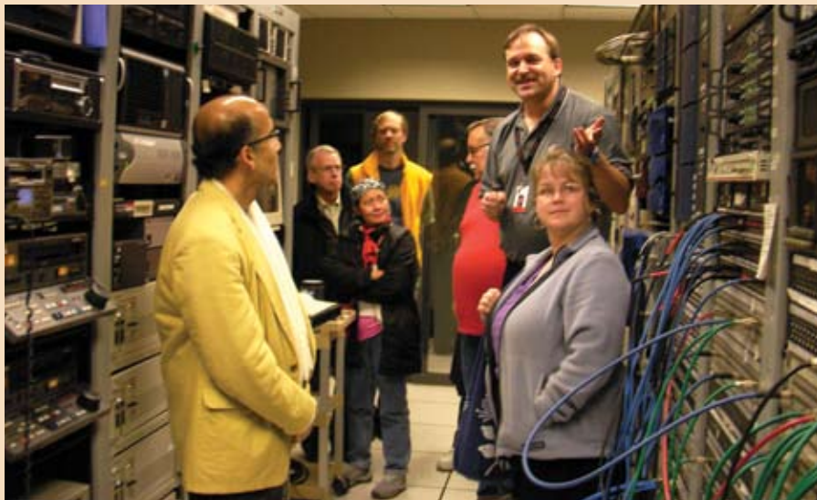
Mike Janes, director of engineering for the Portland Trail Blazers explains the processing needed to provide an HD signal feed to the new large arena screens in the Portland Rose Garden Arena.
