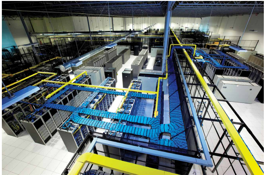
An overhead view of a portion of the server room at the Raging Wire data center facility.
