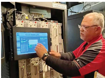
Comark customer service field engineer, Michael Smith, demonstrating the various monitoring display features available on the new WCMH transmitter recently installed in the Columbus plant.
