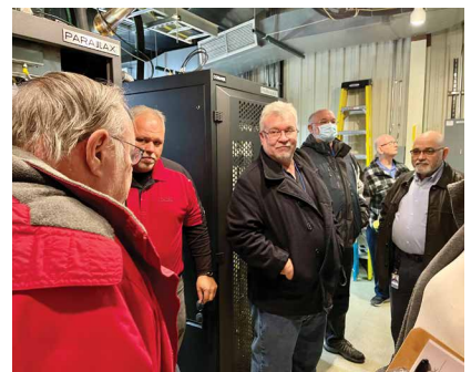
In the center: Ken McCrimmon, WCMH Television chief engineer, conducting the transmitter plant tour in Columbus.
